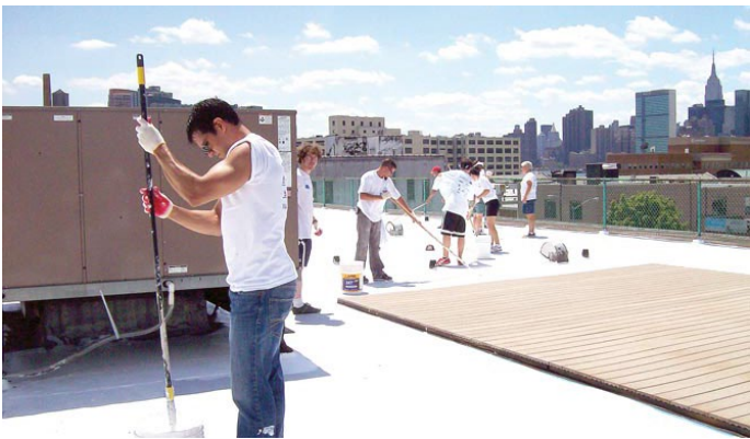
Reflective / cool roofs
